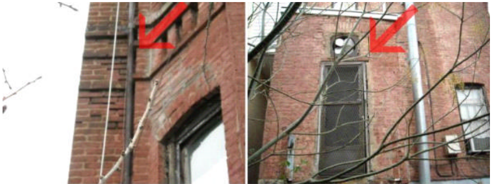
The brick work at the rear kitchen addition needs repair. There is some sporadic tuck pointing that is needed at the side walls.
