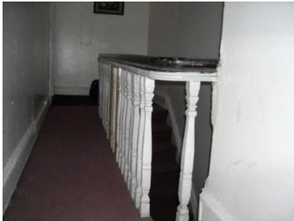
The railing is broken. The balustrade is loose. The rails are too low, not child safe, have broken and loose picket. Rebuilding the rail is needed.
