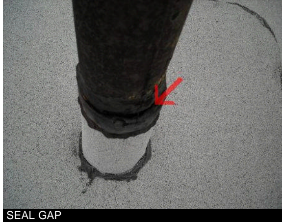
1 Plumbing vent collar needs repair.
