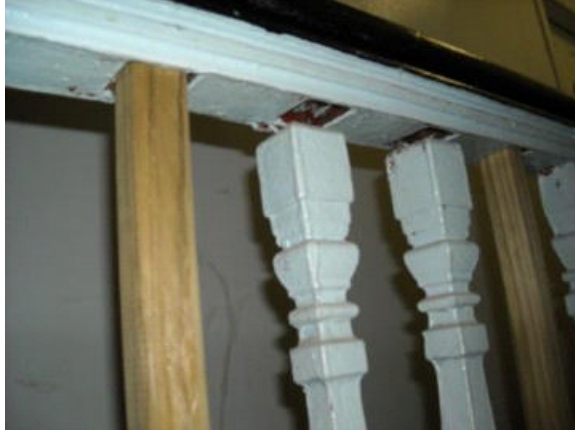
The stairs are narrow. The upper stairs are being supported by an added cross brace.
