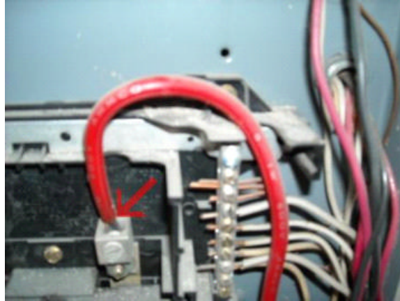
Heat damaged wiring was observed in the panel.
