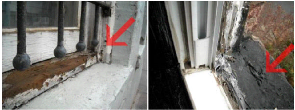
All the wood trim at the windows and doors is in bad shape.
